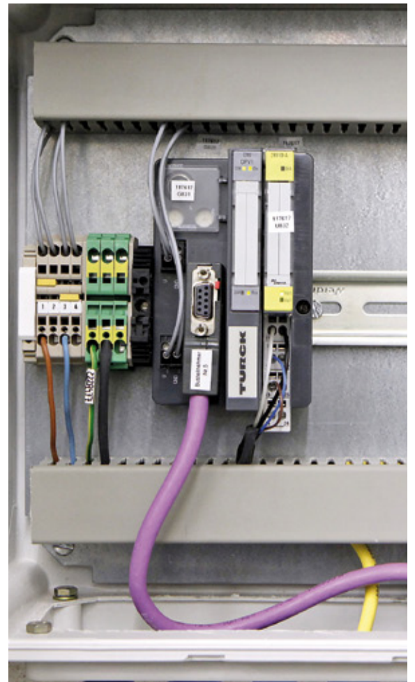
The screen data reaches the PCS7 process control system via Profibus and Turck's BL20 I/O system
